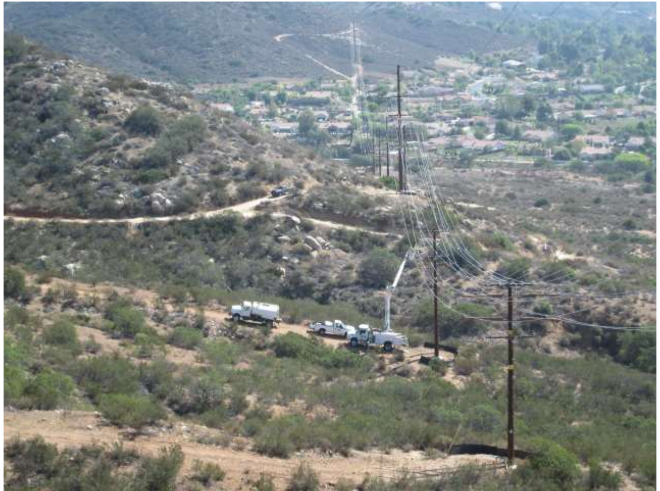
Photo 1: As crews were preparing for wire pulling activities at Location D34, water tenders were staged in accordance with the Project Fire Plan.
