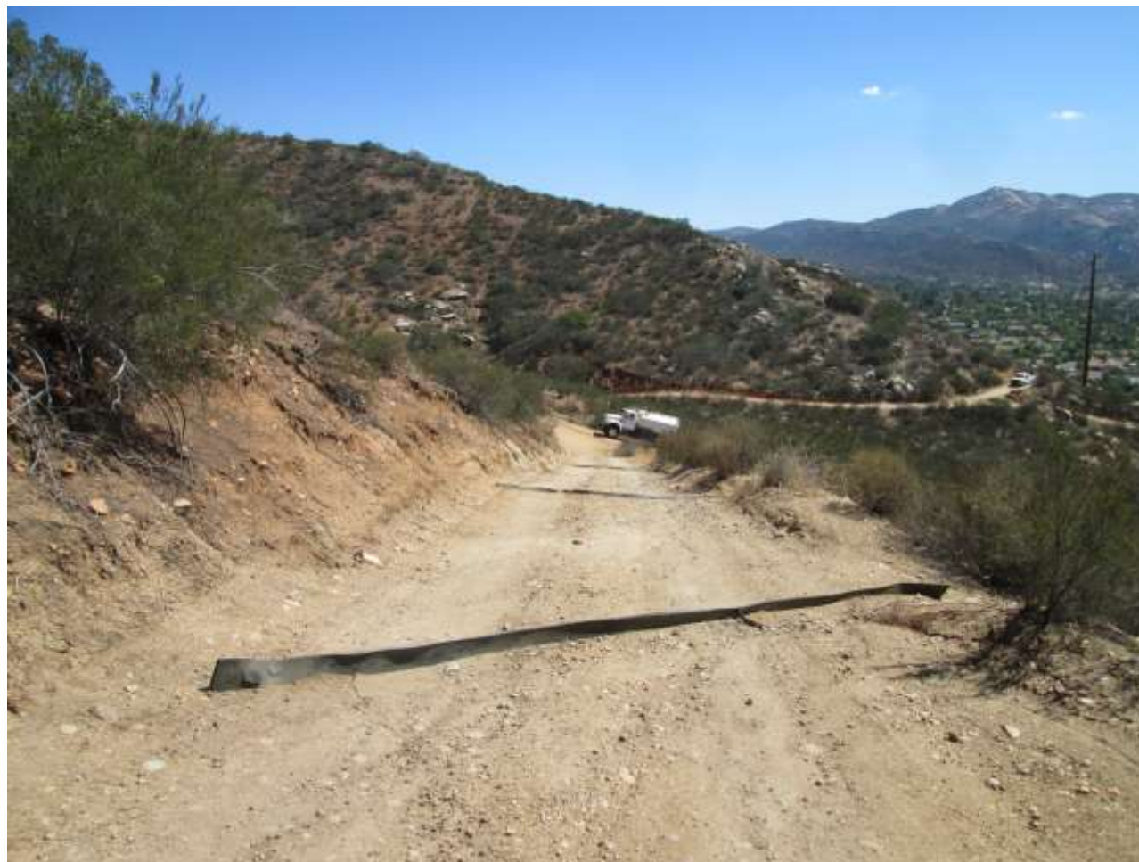
Photo 6: Water bars installed for erosion control along the access road between Locations P32 and D34 were observed in good condition (APM-HYD-1).
