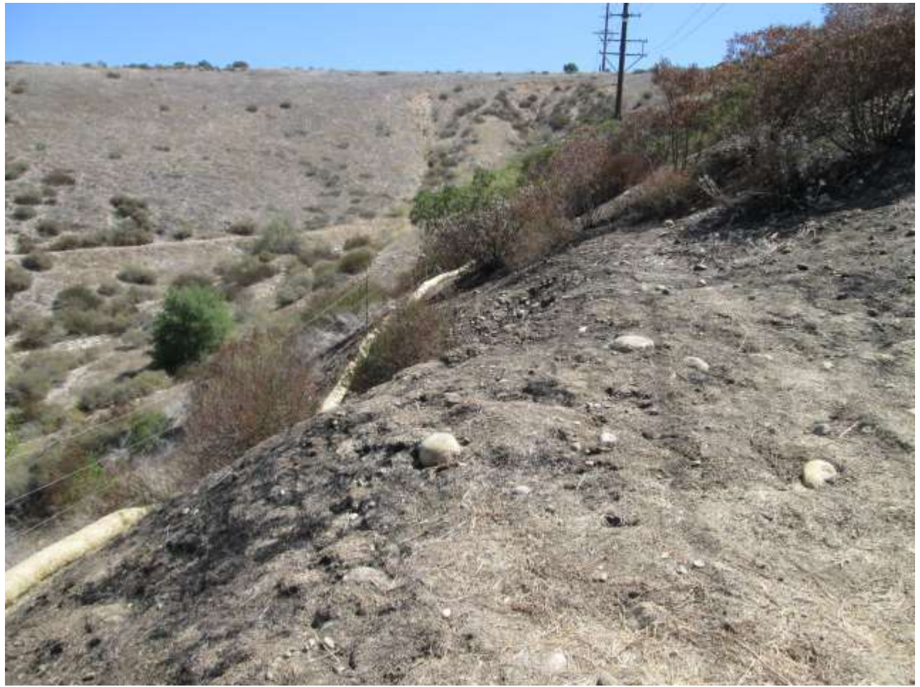
Photo 5: Construction crews installed sediment control BMPs (straw wattles) at the localized burn area (adjacent to Location P22) identified in CPUC WR 014.
