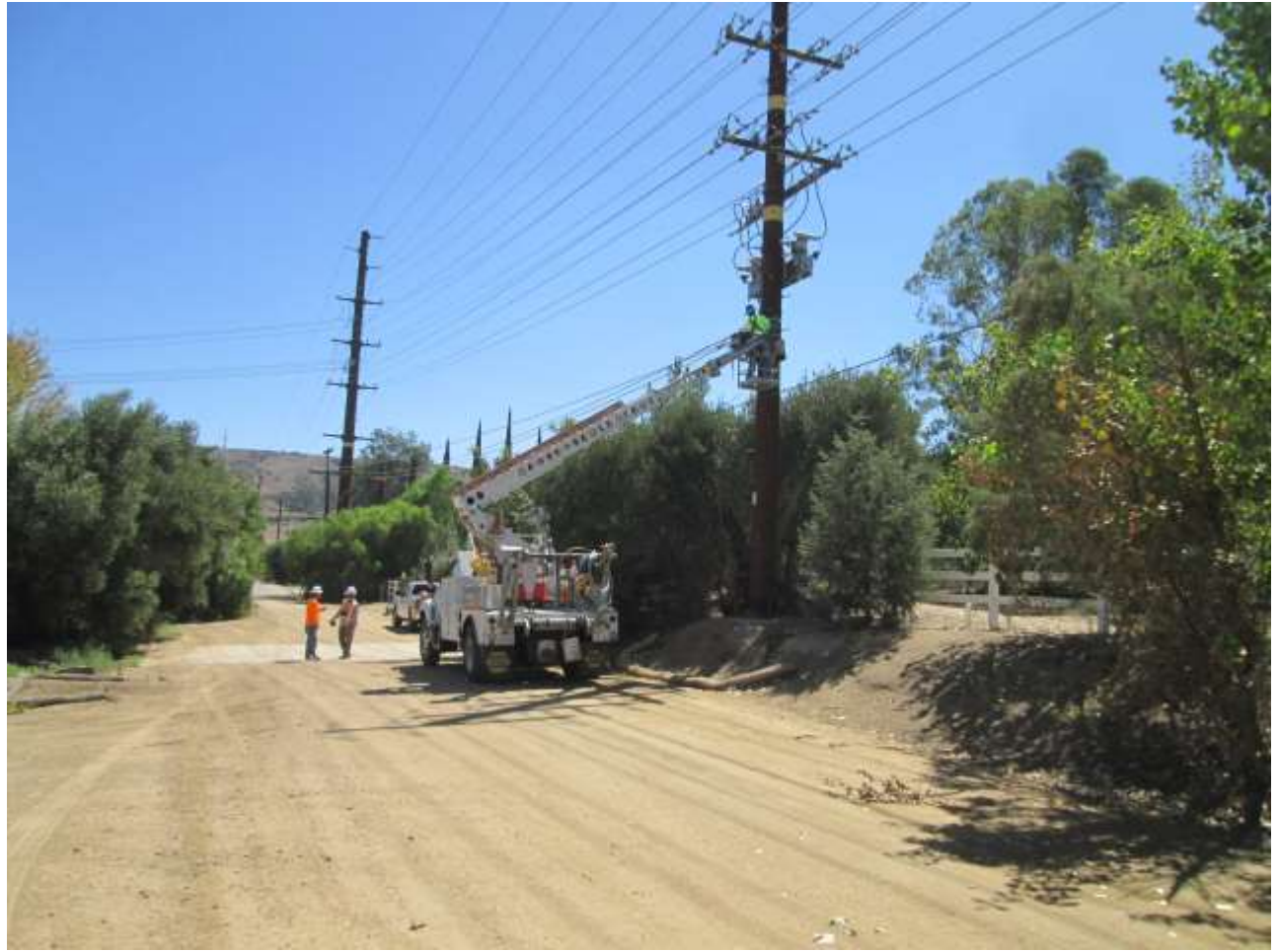
Photo 3: Construction crews were observed preparing for fiber optic installation at Location D7. SWPPP BMPs, such as straw wattles and silt fencing were observed intact and functional.
