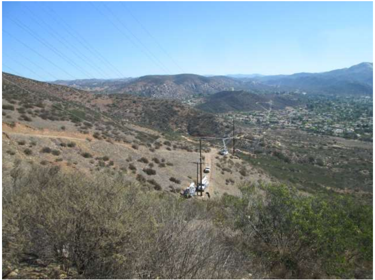
Photo 2: Construction crews were observed staying on approved access roads during wire sagging and dead- ending activities at Locations D31 and D33.
